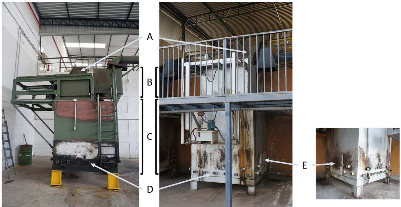
Figure 1 – Oxyclean incinerators with (A): loading ramp; (B) airlock; (C) incineration chamber; (D) nozzle, (E) lateral doors. Left: incinerator in Contagem; Middle and right: incinerator in Santa Luzia.
